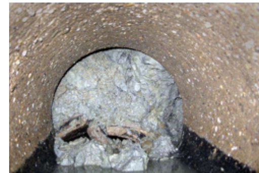
Blockage in Sewer Pipe
